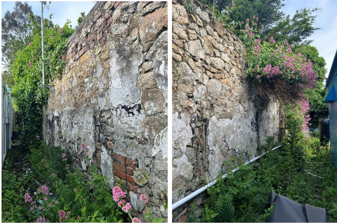
Plate 13,14 View of sections of original wall and later brick sections, with historic lime surfaces evident
